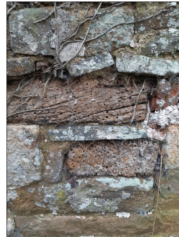
Holes in an old lintel in the south boundary wall are evidence of boring (!) insects
